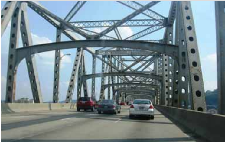
I-71 / I-75 SB Bridge over Ohio River at Cincinnati (Brent Spence Bridge)
